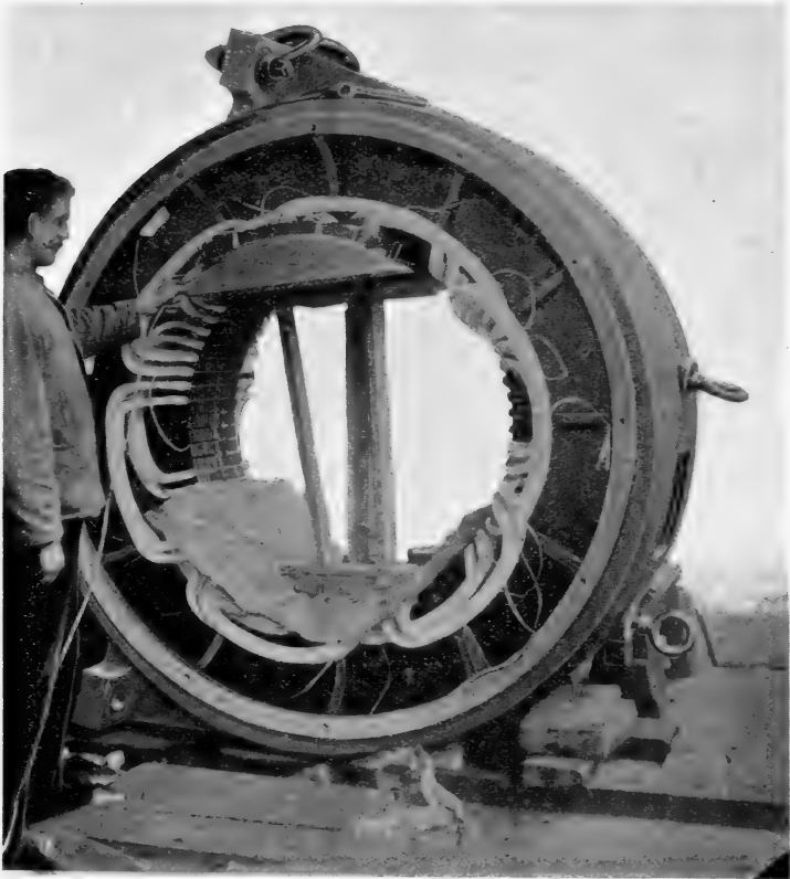
FIG. 372.—Winding Three-phase, Whole-coiled, Double-coil Winding in Three Ranges (Two Ranges completed)—(Bruce Peebles).
